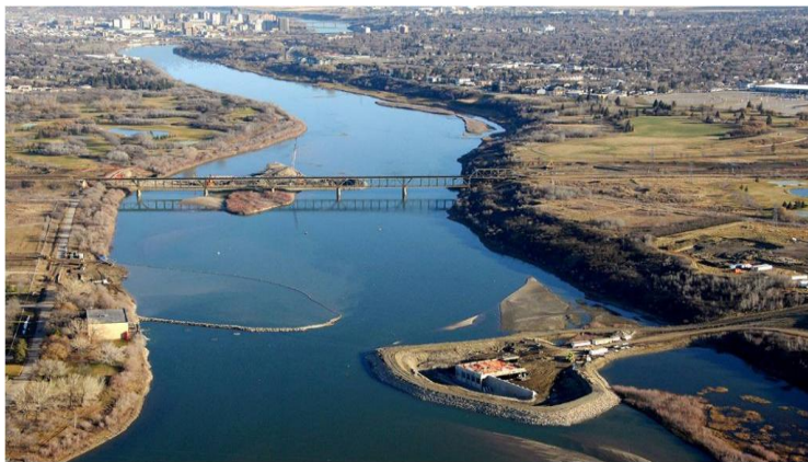
Aerial view of construction of new intake facility upstream of the Queen Elizabeth Power Station.
