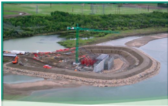
Dams in the river keep water out during construction of the new water intake
